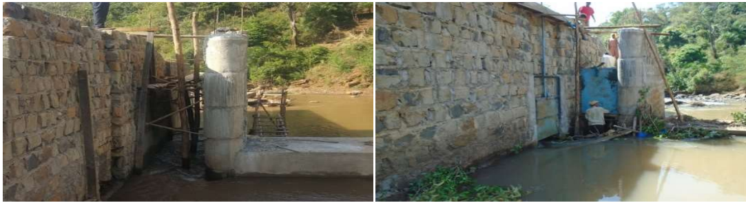
Figure 5: Divide wall constructed b/n retaining wall & weir body and sluice gate fixed
