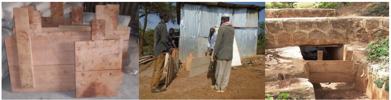
Fig 17: Division box gates fixed into the division boxes slots
